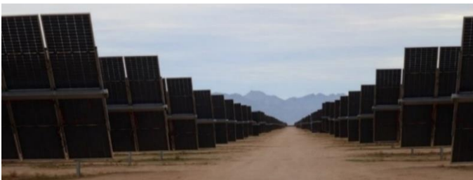
Photo: Sonoran Energy Center, Buckeye, AZ
