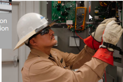
Leander Sansar, Substation Electrician, performs maintenance on the DC system in a substation control house.
